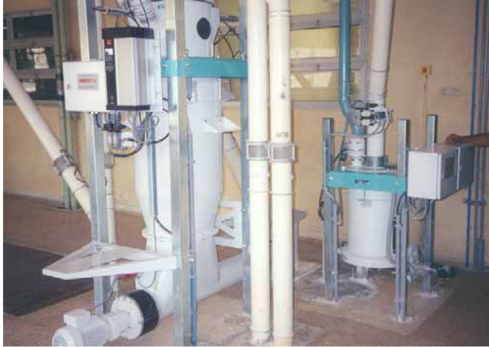
A Flour weighing scale and premix feeder have been installed in this mill in Egypt. The flour scale weighs the flour and the premix discharges using the loss-in-weight principle. The flour and premix is discharged into a mixing conveyor on the floor below
