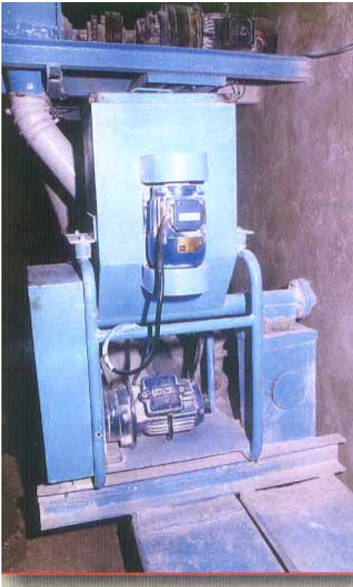
The volumetric feeder equipped with a screw discharge is placed directly above the flour collection conveyor in a mill in India. The premix is fed into the conveyor by gravity.
