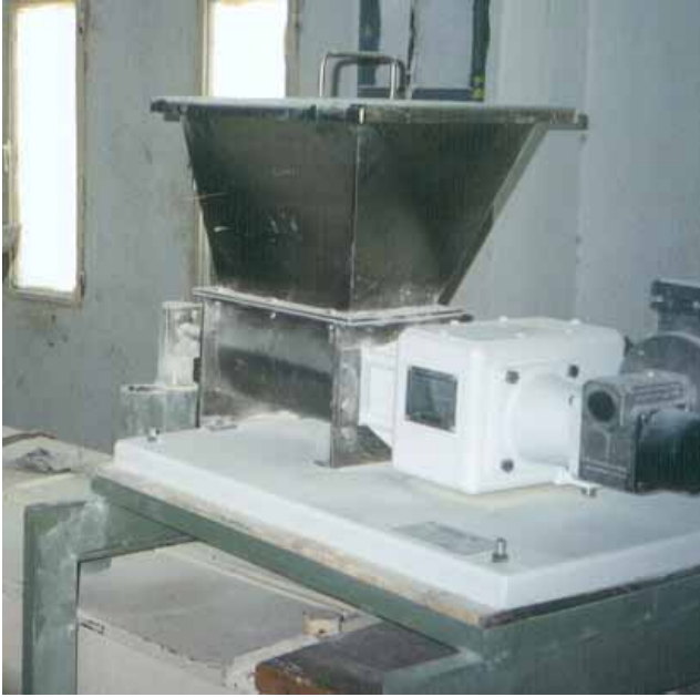
The volumetric feeder is equipped with a screw discharge and is placed directly on top of the flour collection conveyor in a mill in Jordan.
